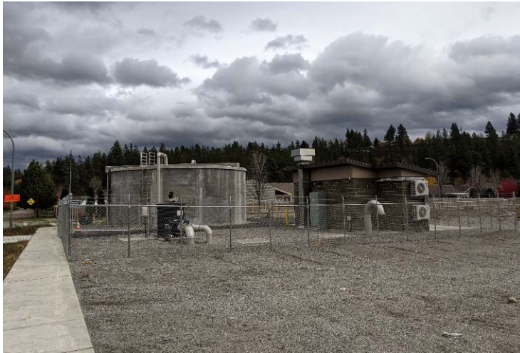
12 th Ave EQ & Lift Station
