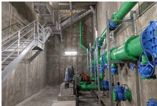
12 Ave Lift & EQ Station
